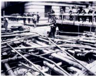
A 1918 photograph of the utilities beneath Wall Street, N.Y. - showing the already congested maze of underground utilities
