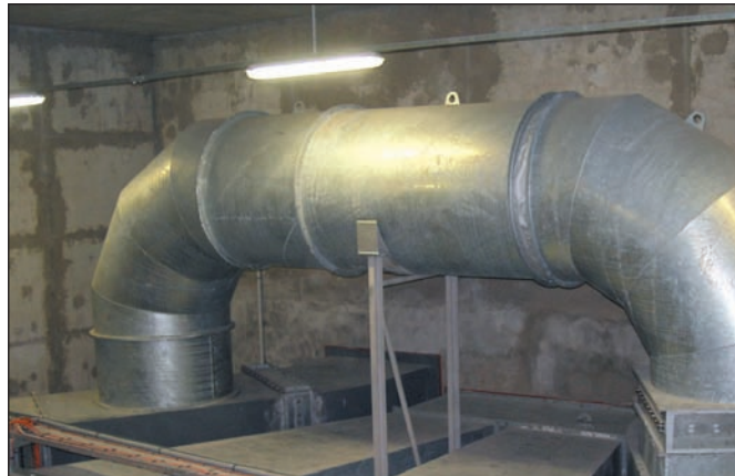
Figure 12 By-pass usine de ventilation nord
